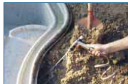
9. Backfilling All around the perimeter wet sand is backfilled under the edge of the preformed pond to fill any cavities.
