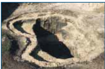
7. Fill-in Adjust the different depths with filler sand until the finished excavation looks like this.
